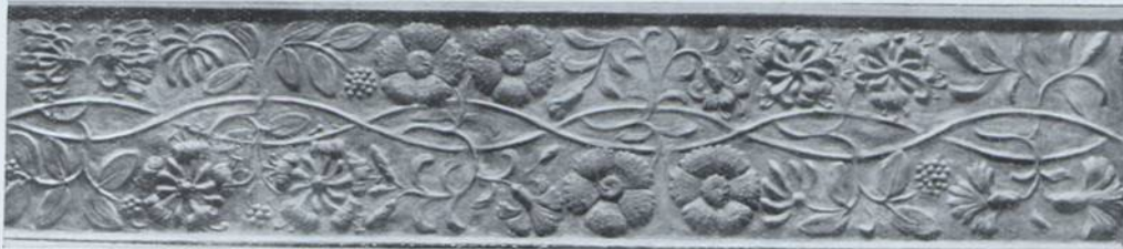
PLASTERWORK—CORNICHE AND CEILING BAND—DESIGNED AND EXECUTED BY A. J. GLOVER, 10, TURLE ROAD, TOLLINGTON PARK, LONDON
