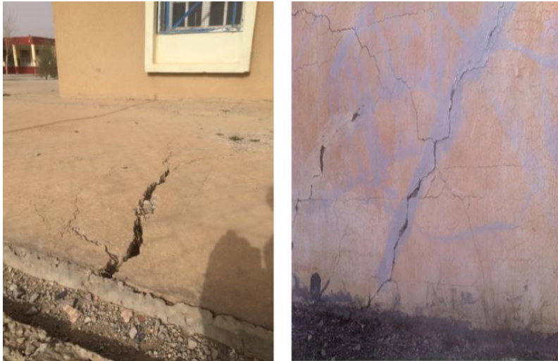
Fig. 1. Structural damages on building caused by expansive soil in Mila region
