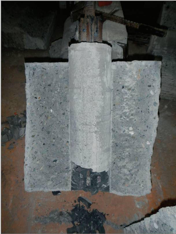
Photo 15. Damaged concrete foundation specimen
