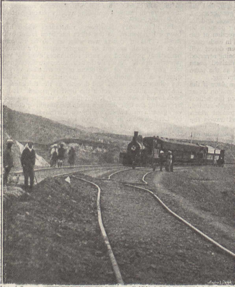
View showing distortion of rails caused by earthquake between Sanzal and Old Chaman.
