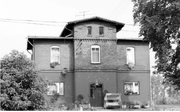
Fig. 2. Lubrza station. The building has been transformed into living quarters. Windows on the ground floor have been rebuilt and all the frames have been ineptly exchanged. The ground floor elevation has been painted (photo: M. Konopka, 2009)
