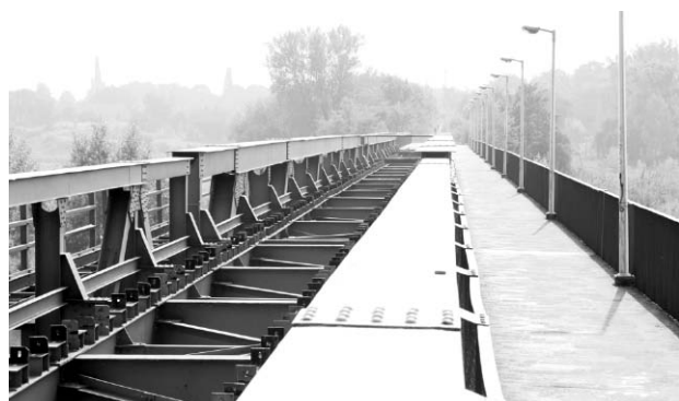
Fig. 5. The pedestrian footbridge on the railway bridge over the Oder between Krapkowice and Otmęt. The track was removed after the July 1997 flood. A pedestrian footbridge has been in operation here since the 1930s. At present the reconstruction of the bridge into a road one is under consideration (photo: M. Konopka, 2009)
