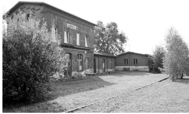
Fig. 3. Krapkowice station. The building is inhabited on the first floor. The ground floor has been unused since 1990. The building is squalid. New and ill-selected window frames in the flat are explicit (photo: M. Konopka, 2009)
