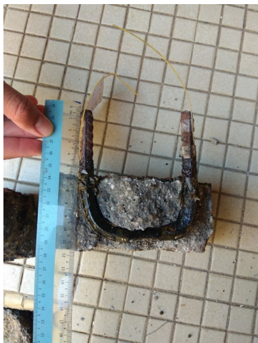
Fig. 3. The concrete sample was hacked with exposure of the steel bar.
