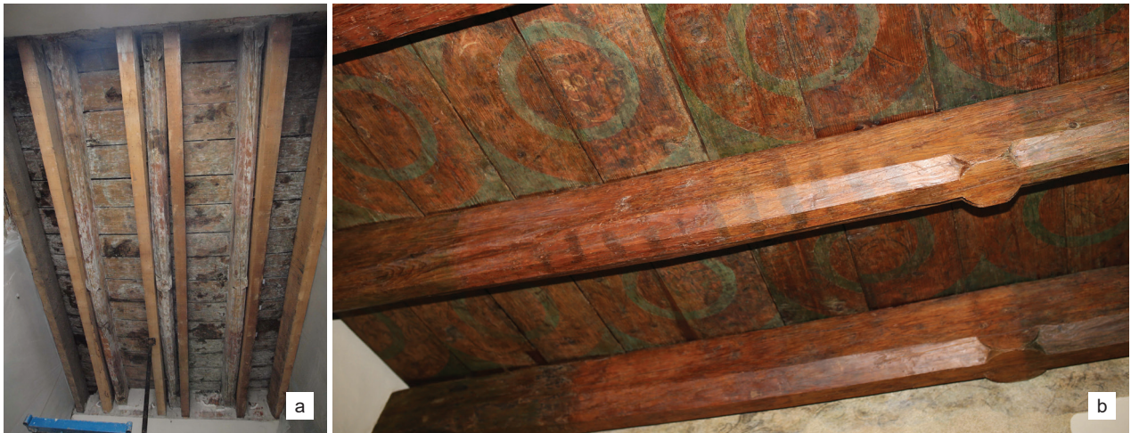
Fig. 7. Dominican priory in Krakow – Late Gothic wooden beam ceiling (“lower” one): a) while uncovering, b) after building and conservation work completion (photo by A. Luboń-Radwańska)
