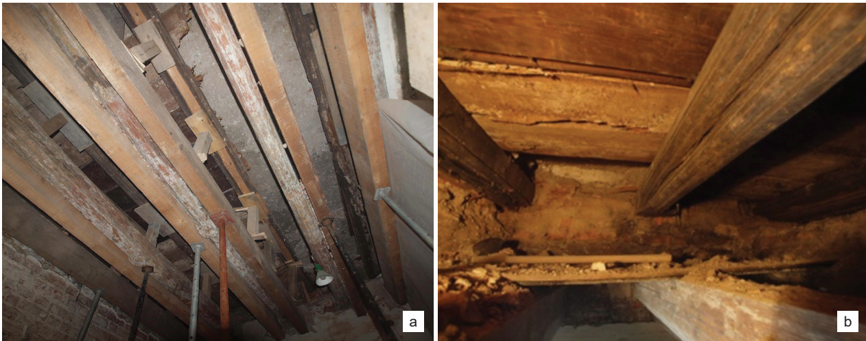
Fig. 8. Dominican priory in Krakow – wooden beam ceiling (“higher” one) – “technological”: a) both ceilings while exploring with intervention support, b) rubble charge filling the space between the ceilings (photo by A. Bojęs-Białasik)
