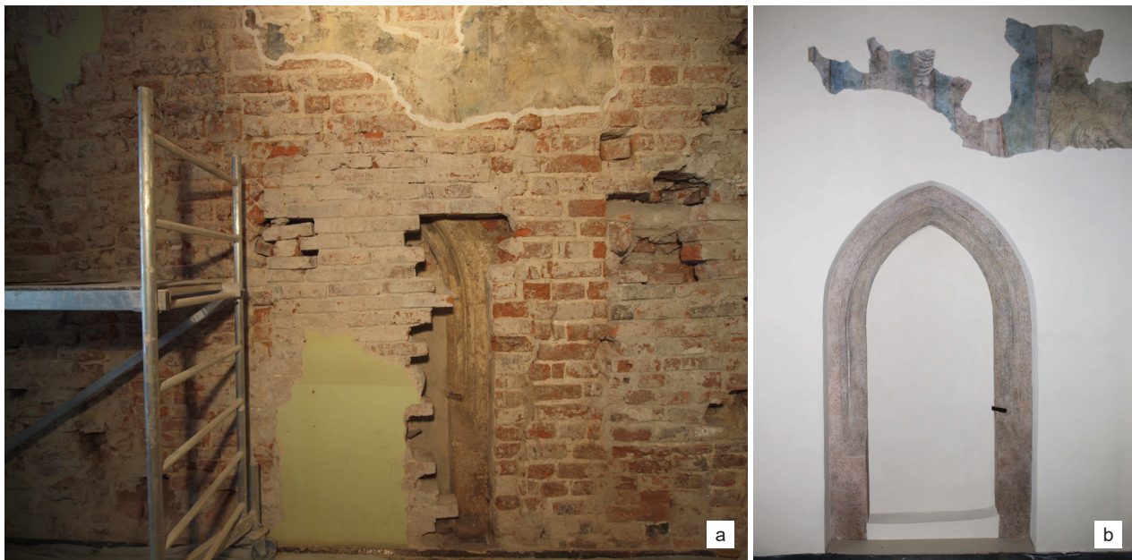
Fig. 6. Dominican priory in Krakow – the eastern wall with a brick covering and a fragment of polychrome above it (Crucifixion?): a) gothic portal while uncovering, b) gothic portal and polychrome after conservation work completion (photo by A. Luboń-Radwańska)
