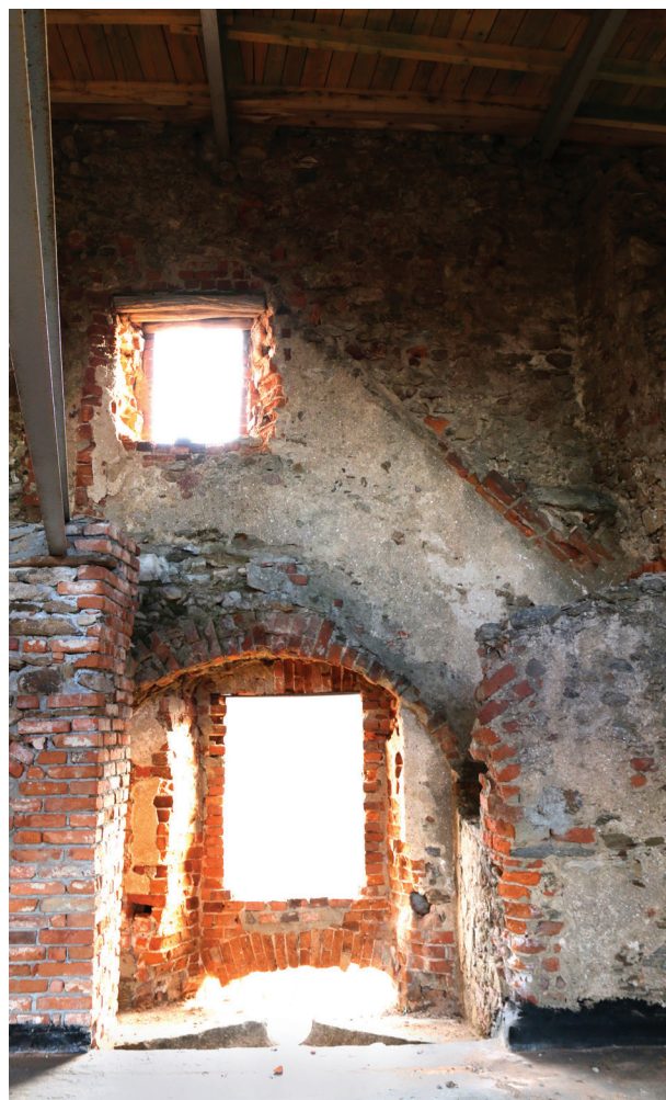
Fig. 15. Grodno Castle. The outline of plaster on the wall shows the flight of stairs leading to the porch (photo by M. Chorowska)
