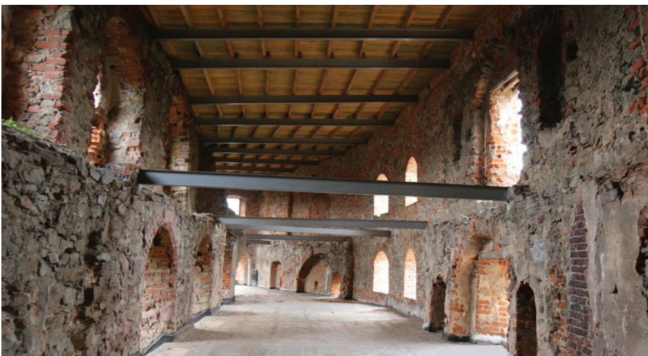
Fig. 14. The interior of the southern wing from the east, during construction works in 2019. To a large extent it corresponds to the lost knight's hall, which, like today, was of two storeys height (photo by M. Chorowska)
