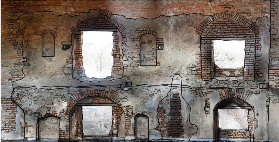
Fig. 13. Grodno Castle. Window openings, niches and nests in the northern wall of the southern wing, photo-scan outlined (elaborated by R. Biel)
