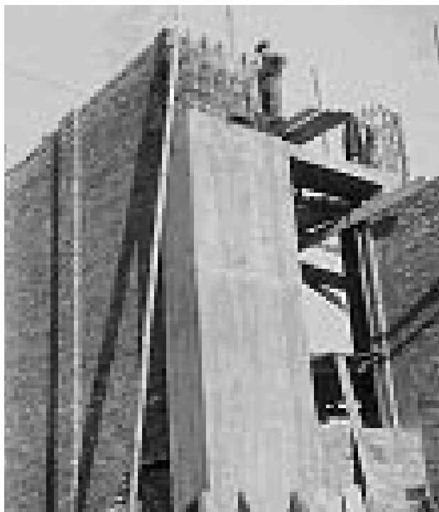
Fig. 2. Building church walls, in the foreground we can see a reinforced concrete column [1]
