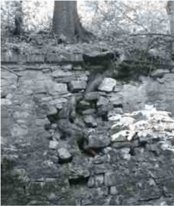
Fig. 17. Destructive influence of plants on the construction structure (photo: J. Potyrała)
