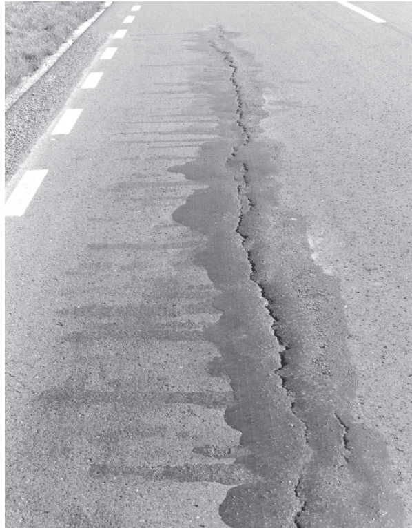
Figure 1: Longitudinal crack in the surface as a result of uneven settlement of the embankment.
