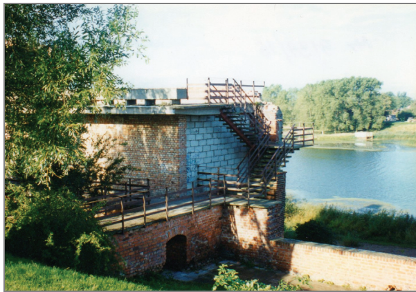
Fig. 2. The Latin School after its partial restoration in the 1970s (photograph by Z. Duda)
