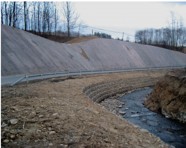
Fig. 14. Landslide in Szymbark after partial stabilization
